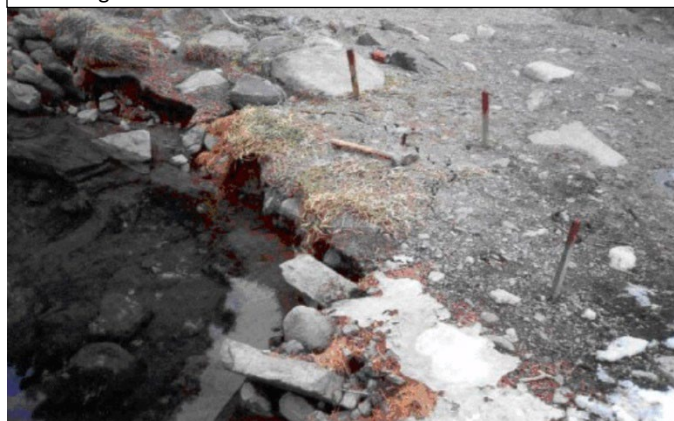
Cracking at the embankment dam crest above the sinkhole. 8
